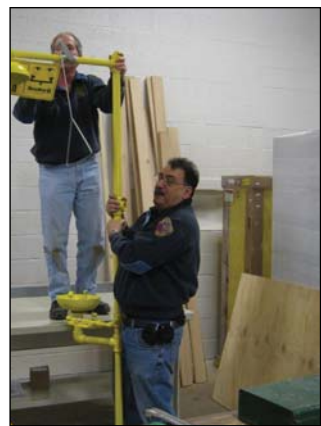
Dan Imfeld and Julius Leone installing drench shower in the HAZ-Mat section of Station 7
